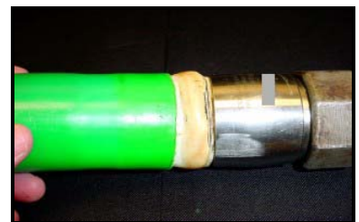
Flexible piping is bulging
