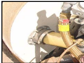
Sump penetration seals in good condition
