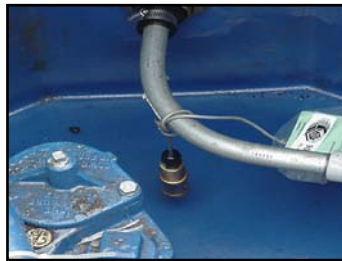
Liquid sump sensor
