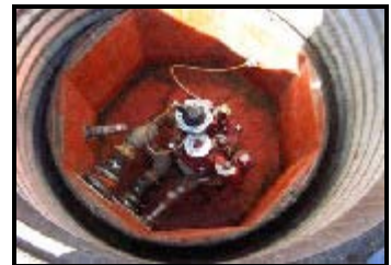
Contained turbine sump
