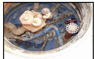
Flexible piping is kinked
