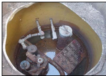
Contained sump with liquid and debris
