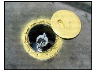
Circular spill bucket lid pulled back to show the fill port with a spill bucket
