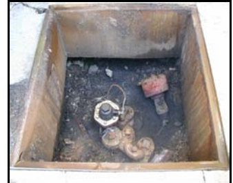
Uncontained turbine sump
