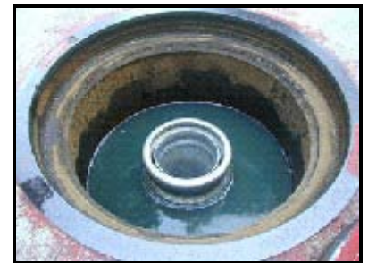
Spill bucket that contains liquid
